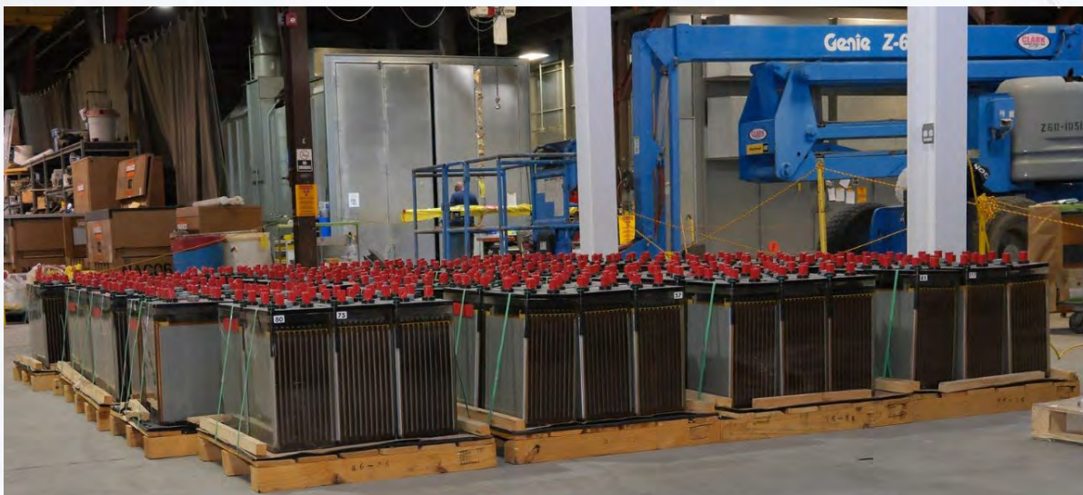
Station backup and industrial cells, surveyed for release at the WCS Alaron Facility.
